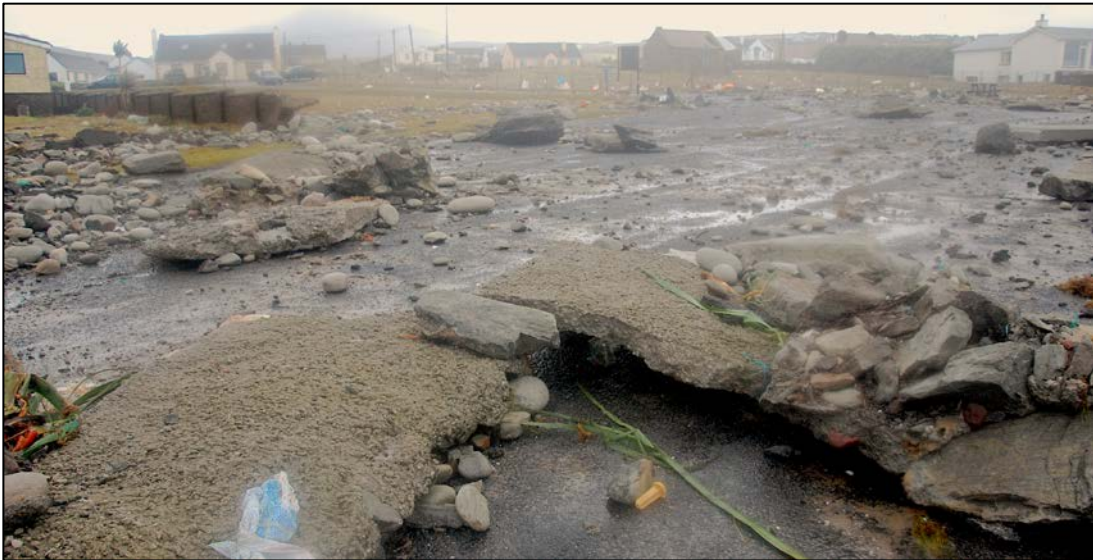
Storm damage Achill Island, Mayo (Photo by Roisin Lavelle)
